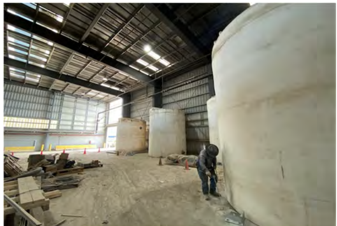
Slurry storage tanks and loadout piping
