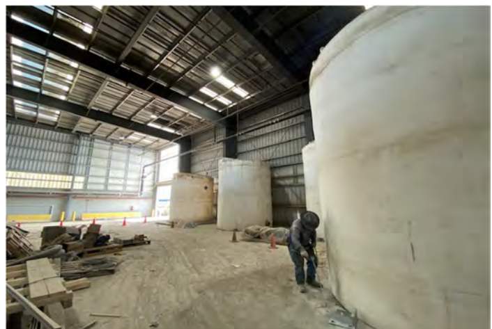
Slurry storage tanks and loadout piping
