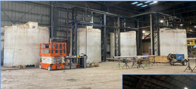
Picture Above Three new (3) liquid holding tanks (right side) have been installed in the transfer station to store processed organic slurry...ready for tanker-truck load out. Note agitation units on top of each unit to keep solids from settling prior to loadout. A fourth tank (left side) has been installed to store recycled water from WWTP for organic
