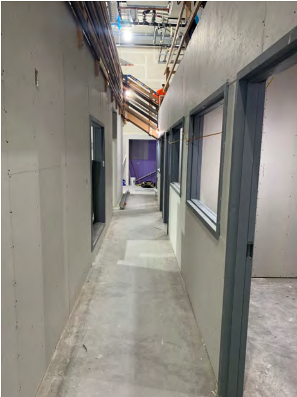
1st floor main hallway view from front door with three hard offices on the right
