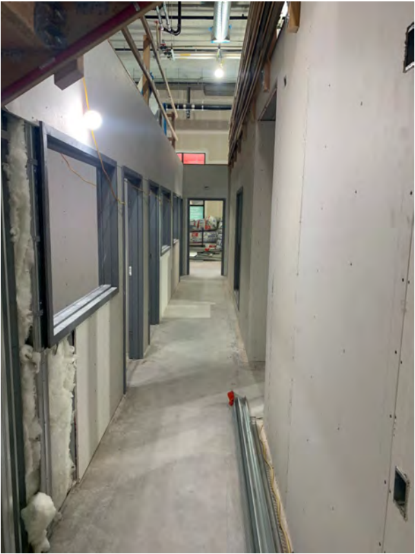
1st floor main hallway view from back with three hard offices on the left
