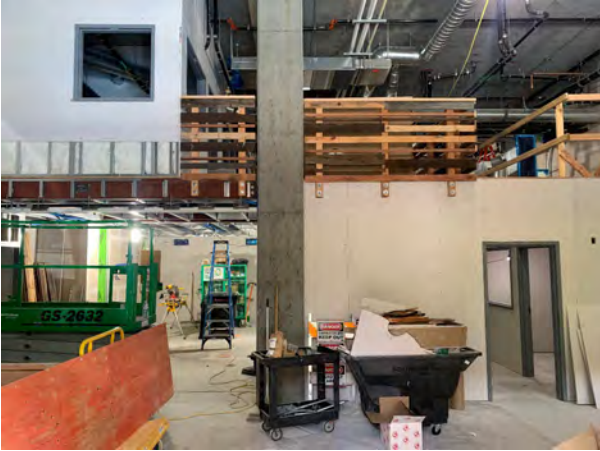
1st floor lobby looking into main conference room (right) and 2nd floor at top left
