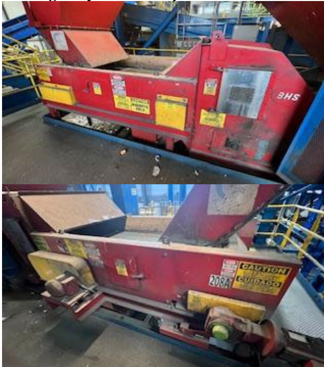
Existing Eddy Current Separator
