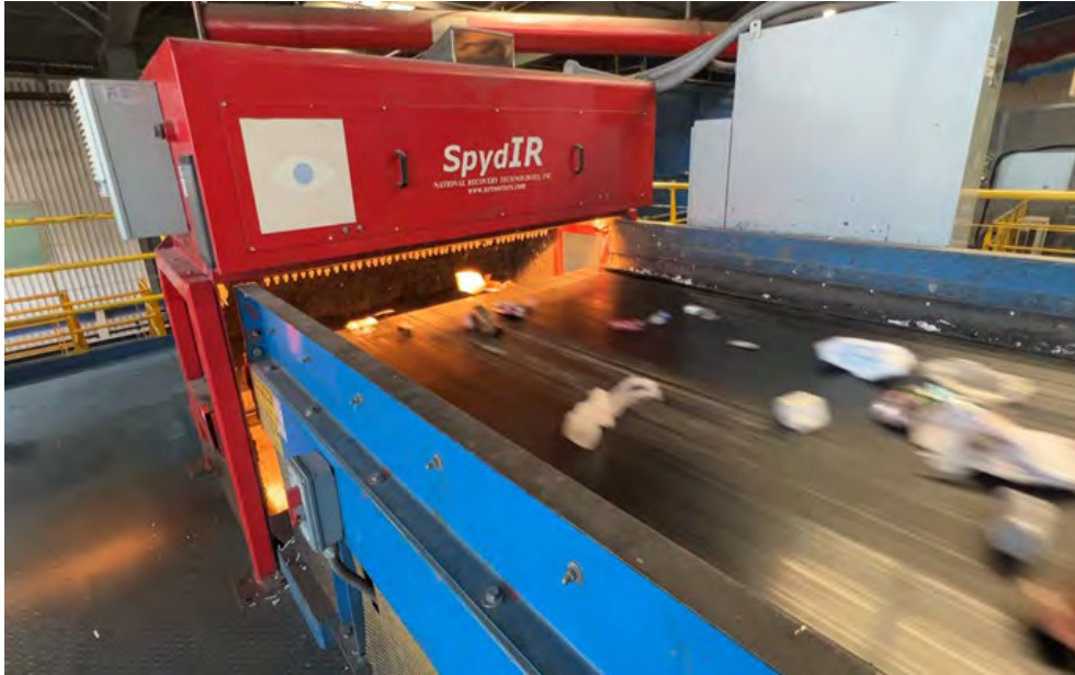
Figure 1 Example of Current Optical Sort Unit at Shoreway to be Replaced
